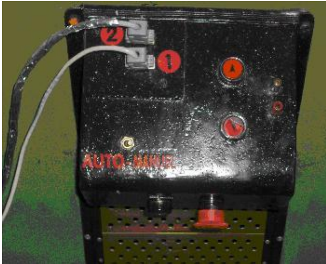
Fig. 1. Control Panel of Forging Press
