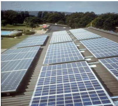
Picture 1 Photovoltaic cells.
